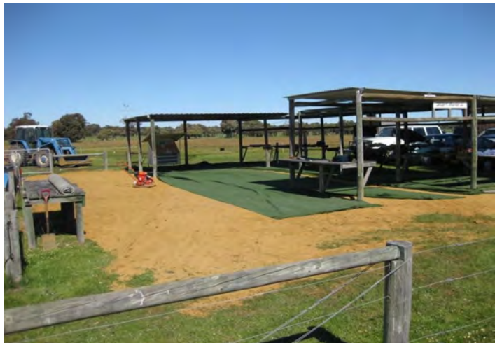
First sections of carpet in place. Concrete surface has certainly saved a lot of work since it was installed in 2015.
