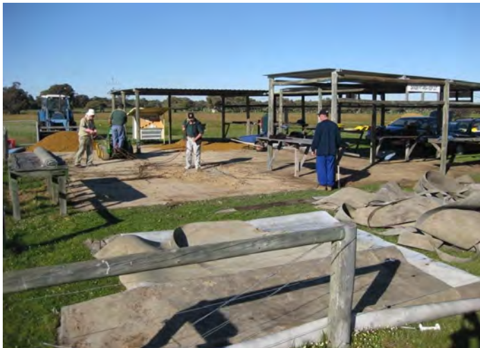
Upgrading the pit floor surface 2009, once levelling completed bowling green carpet was installed
