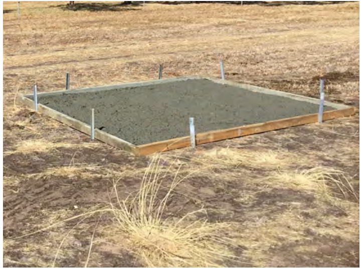
The completion of the helicopter pad, it is obvious it increased in size due to a bit more concrete being left over for the final runway pour.
