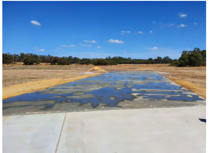
The last section on the northern end of the runway prepared ready for the plastic sheeting and reinforcing mesh to be installed.
