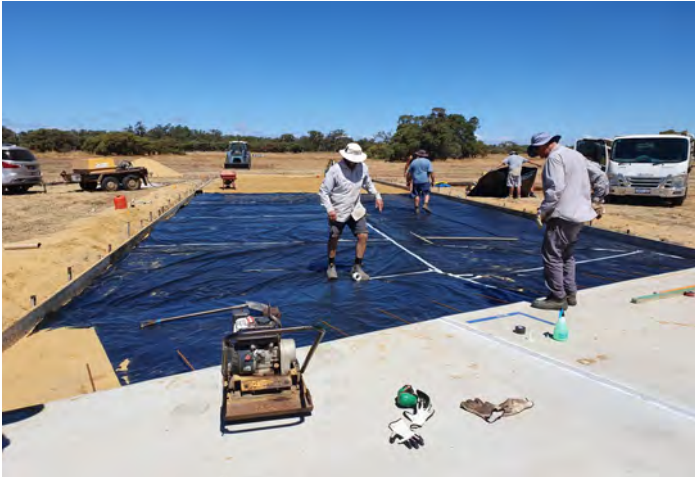
Progress on the second day of the runway project with the plastic sheeting being put in place
